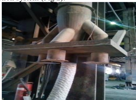
Figure 2) The central local exhaust suction system
